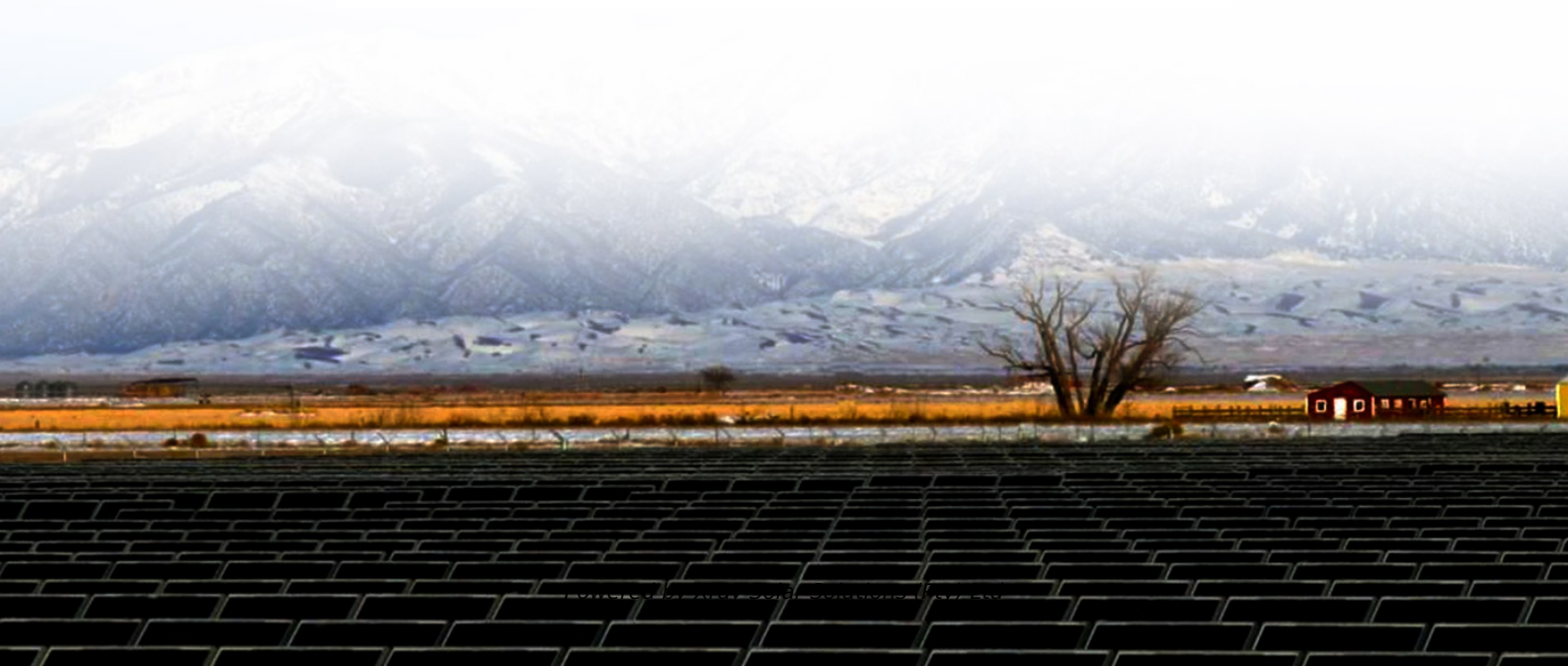
200kWh Battery Cluster
