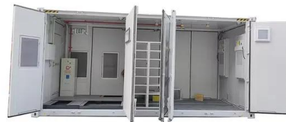
1075KW HH ESS
