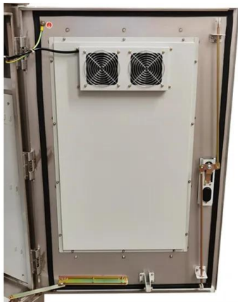
Sarajevo base station communication backup power supply
