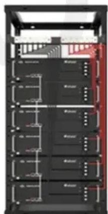
Cabinet and rack installation display
